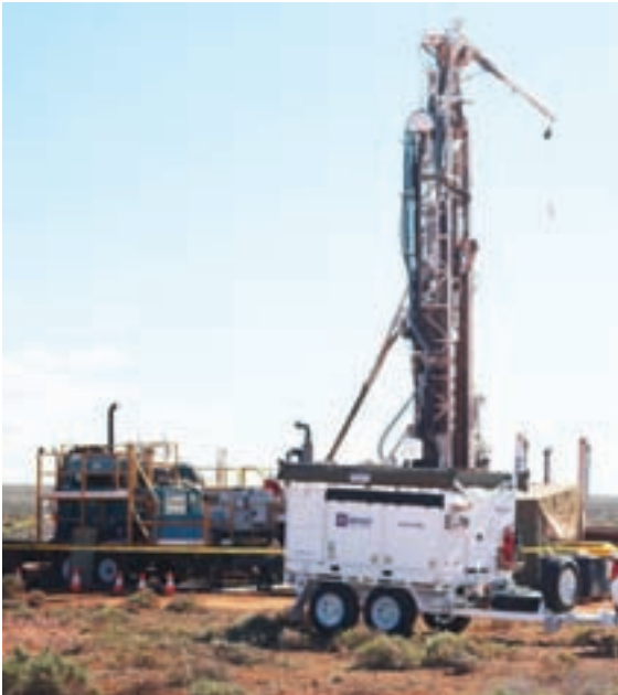
Reflex Lab-at-Rig ► ascertained simply by being on-site. All the work is documented and a report is produced for the client," says Evans. on site in South Australia
